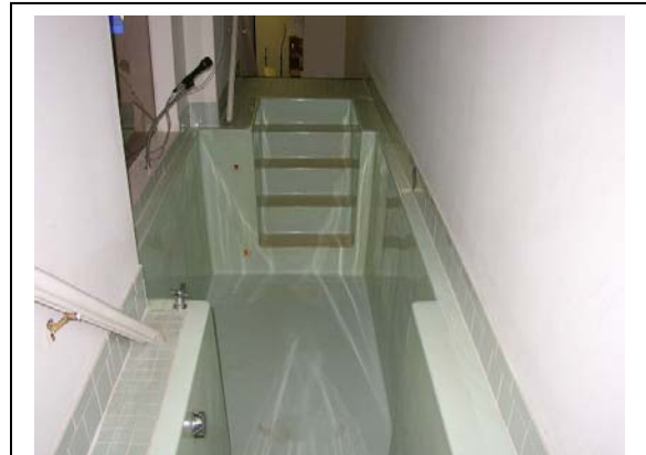
This photo illustrates a corded microphone installed in the baptistery. The risk of electrocution is present for anyone in the baptistery who could contact the microphone. The microphone in this photo should be relocated and suspended from the ceiling or replaced with a cordless microphone.
